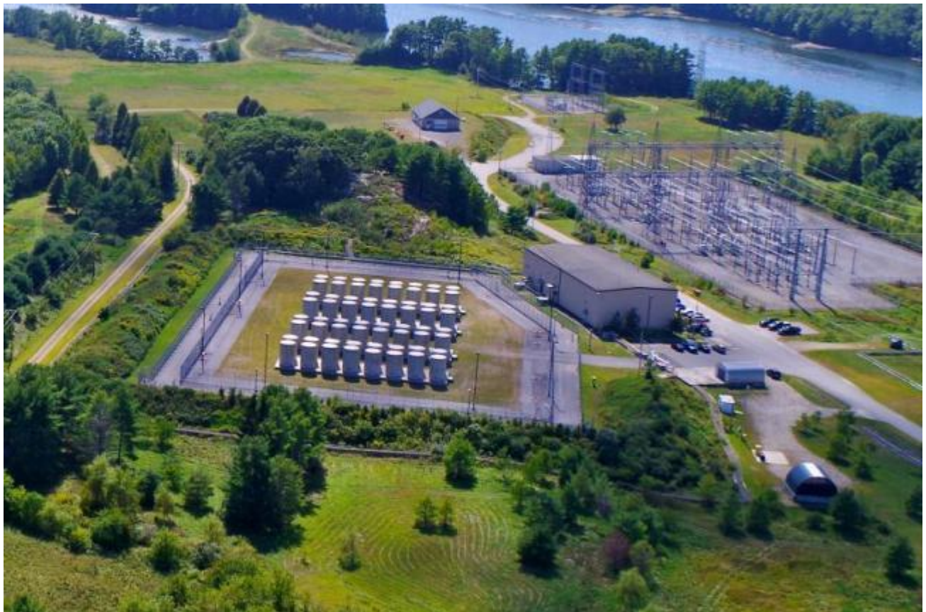
Aerial view of Maine Yankee's Independent Spent Fuel Storage Installation (ISFSI) located on Bailey Point, Wiscasset. Courtesy of Maine Yankee
