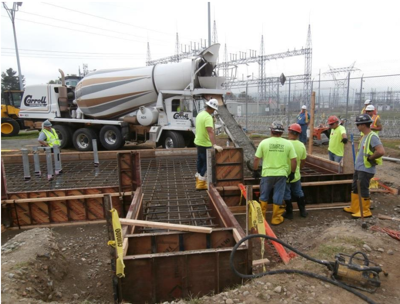
New 200 kW EDG Foundation
