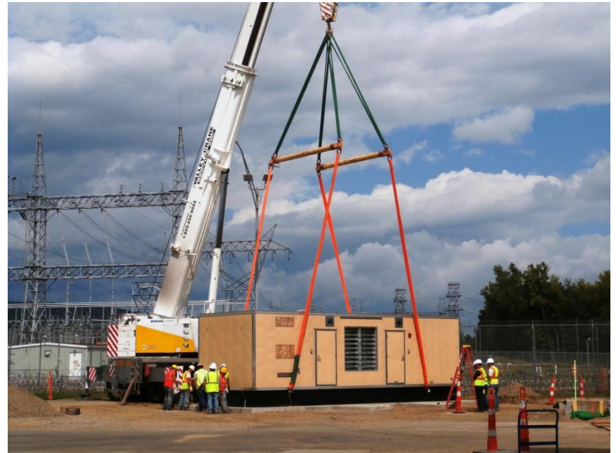
New 200 kW EDG Enclosure
